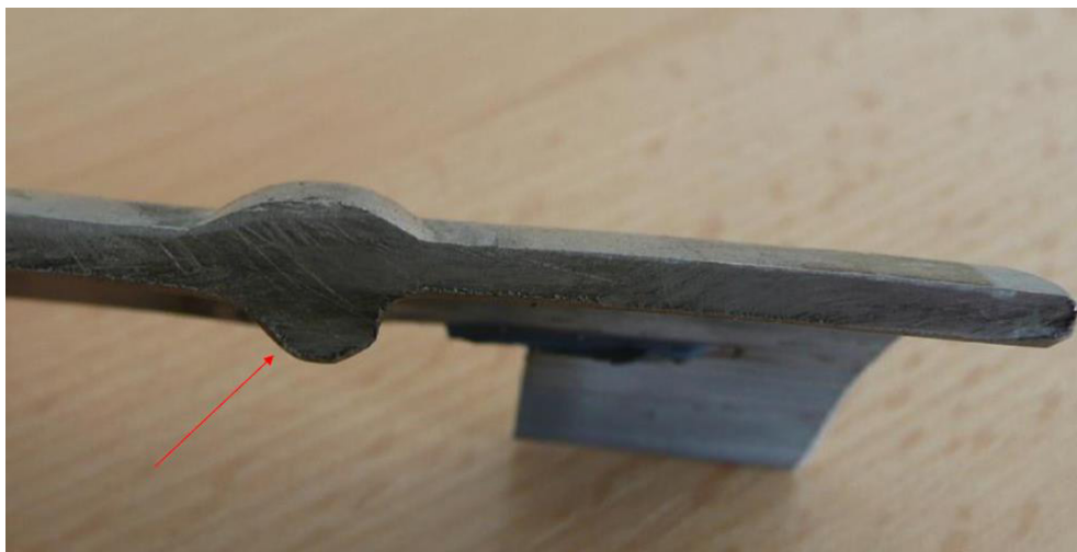
2: Internal protrusion in root of weld
