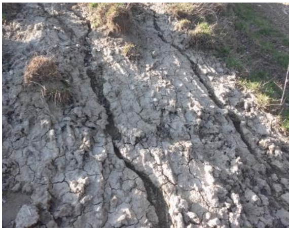
Figure 5 Formation of water erosion on the road
