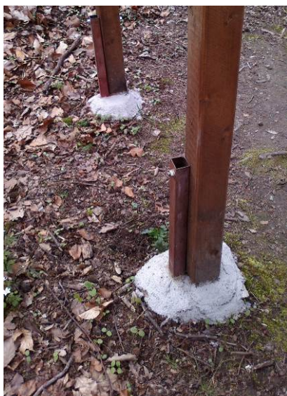
Fig. 3: Inappropriate anchoring of the wooden posts of the information board, structural protection is not ensured (Kotásková)
